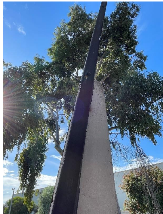
Righthand side of the 1924 Stobie pole showing one of the steel beams.
