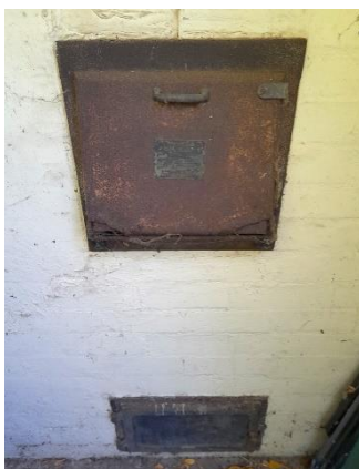
Incinerator furnace and ashpan doors
