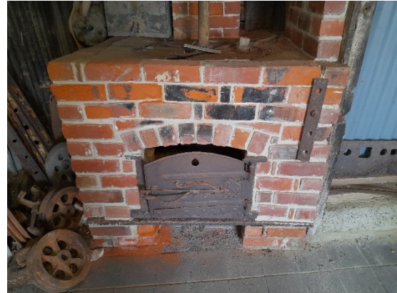
Furnace and boiler feeding steam box.
