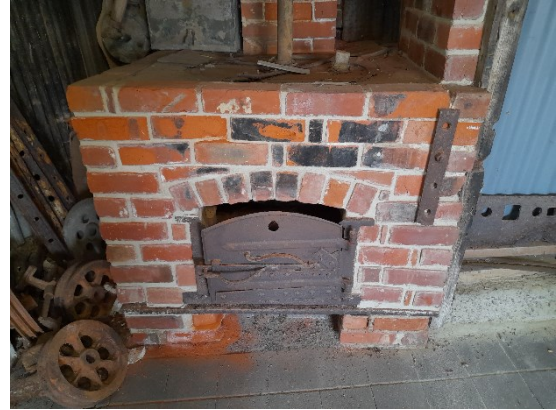
Furnace and boiler feeding steam box.
