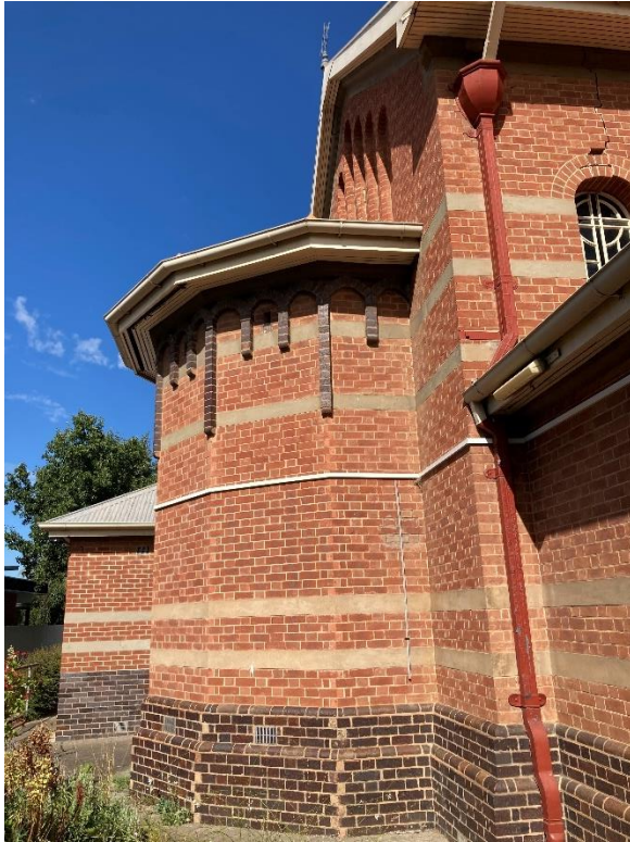
View of details to apse. Note rain head and cracking above the first triple window above the vestry.
