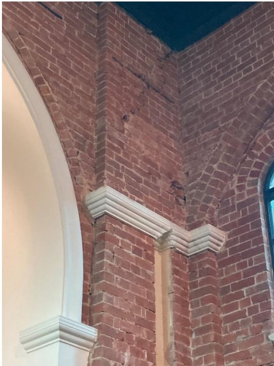
Detail showing the condition of the brick-face after removal of plaster in transept.
