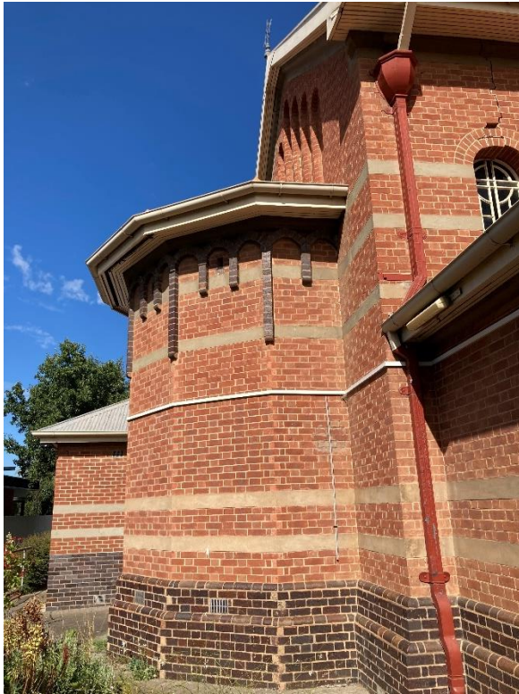
View of details to apse. Note rain head and cracking above the first triple window above the vestry.
