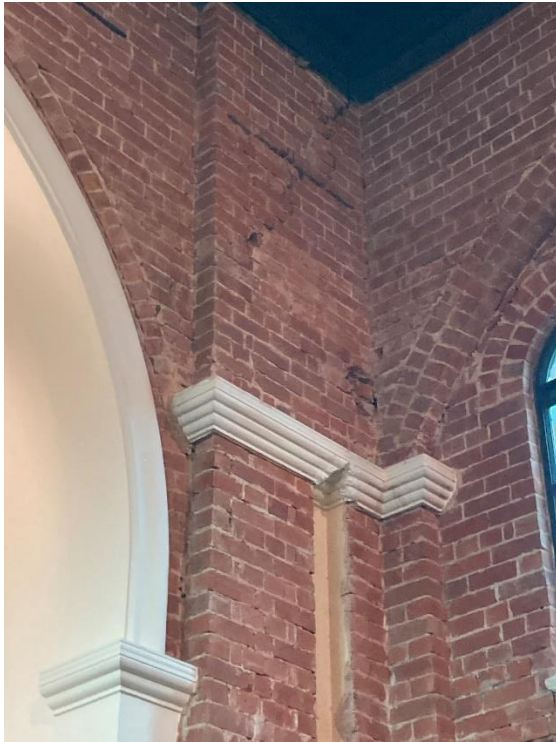
Detail showing the condition of the brick-face after removal of plaster in transept.
