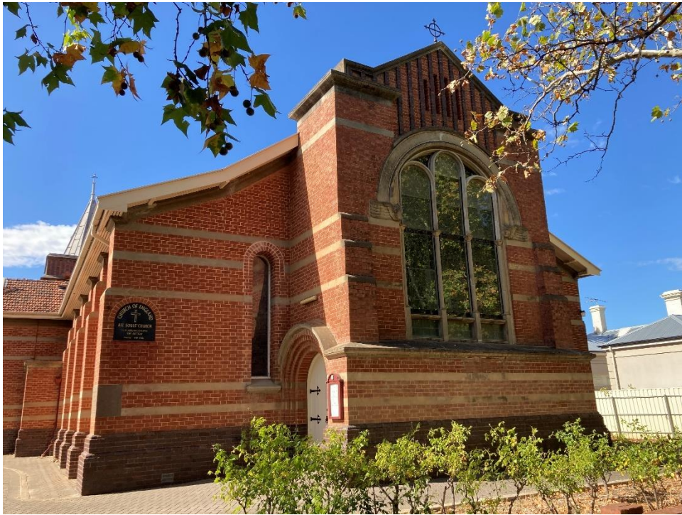
View showing the east window and detailing to narthex. Note stepped surrounds to doors, cement bands, and vitrified brick to gable.
