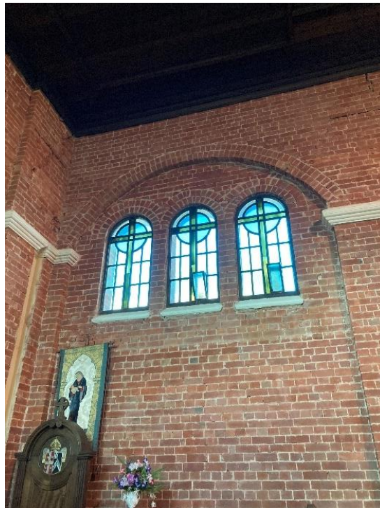
Lead light in the triplet windows. Note the poorer condition of the brick face due to the removal of the plaster from this part of the church.
