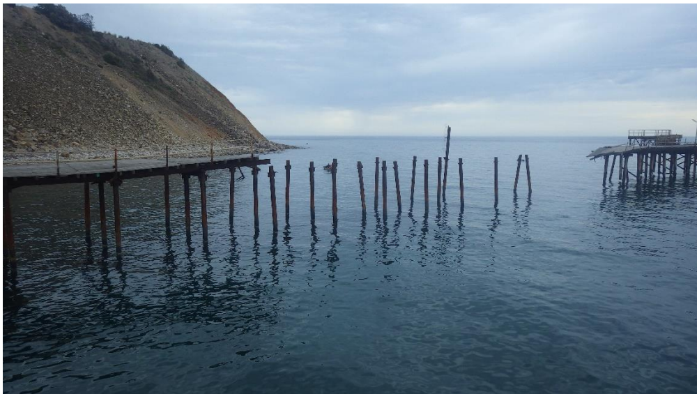
Figure 4B: Old Rapid Bay jetty in December 2018, showing collapse of decking, and severe corrosion of metal piles. Image: © J. Baker.
