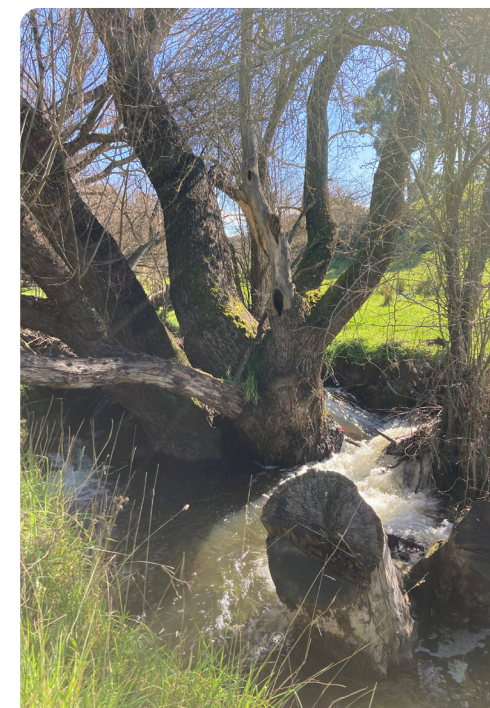
Bank scour caused by invasive willow trees
