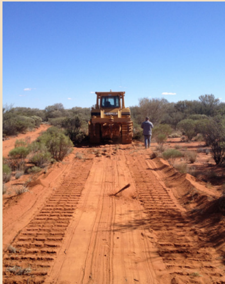
Above: Dozer driver Mark Frahn heading off to work Below: Donald Grant discussing work with Mark
