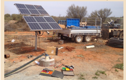
Solar panels set up to power the bore pump
