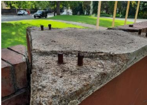
Reinforced concrete base of toppled spire
