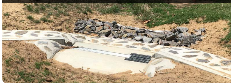
The gravity device inlet built on the Lynch property.
