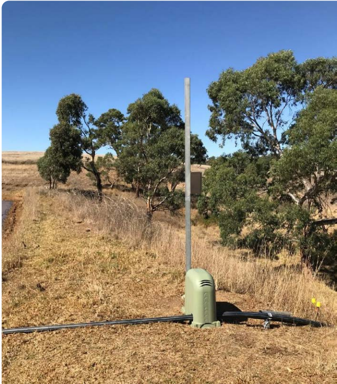
Solar powered pumps are used to release the low flow component that is recorded from the V notch weir.
