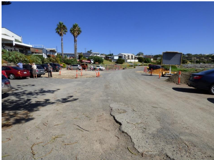
Franklin Parade prior to completion of the carpark Note location of the fenced well area towards the end of the carparking area. 17 March 2017 Source DEW
