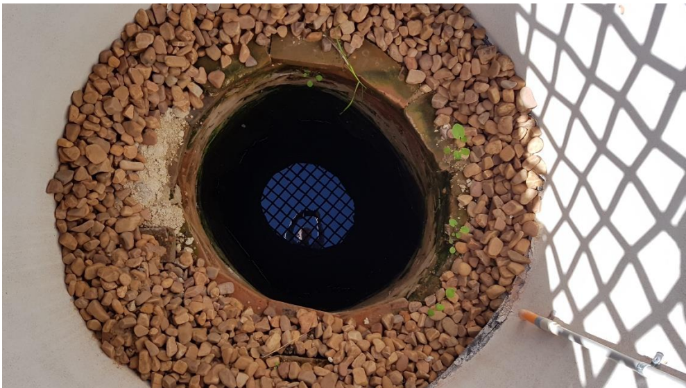
Inside the well 17 September 2019 Source DEW
