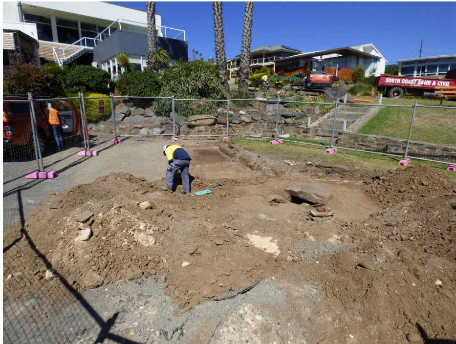
Well site during its discovery and archaeological survey. Note well location directly in front of the Whaler's Inn Restaurant 17 March 2017 Source DEW
