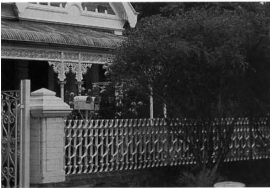
The Hume panels in this Norwood fence have been used to replace cast iron.
