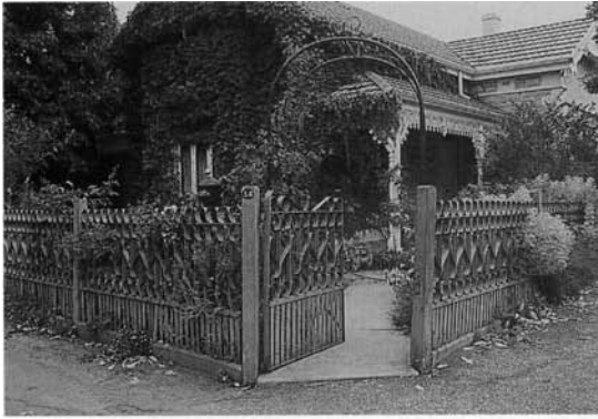
An intact Hume steel ribbon fence in Unley. Rusting and deterioration are unfortunately in evidence.
