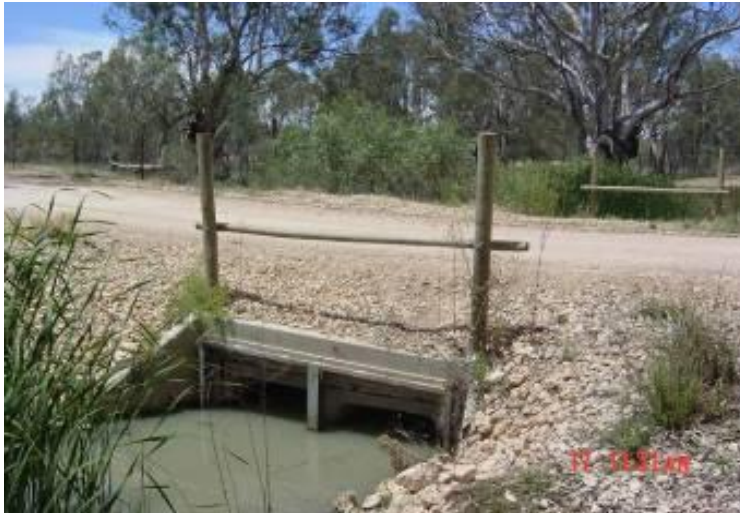
Figure 4: Cosy Corner inlet structure
