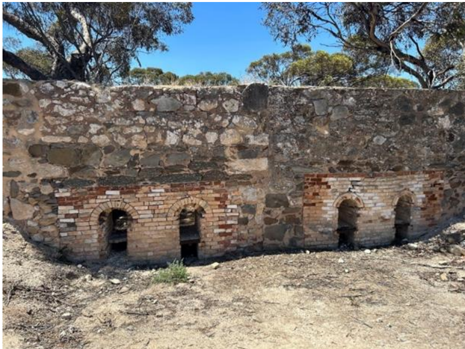
The D-type lime kilns built by George Green in the late nineteenth century.
