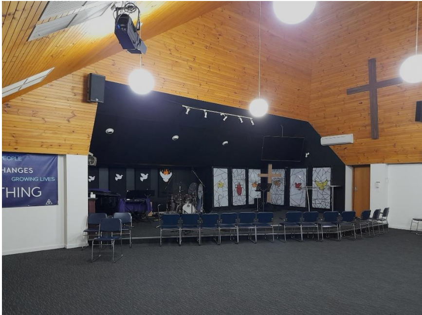
Interior of worship space showing former choir transept, note gyprock glued over face brick and black cloth stapled to ceiling
