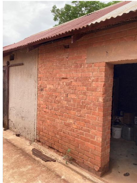
Brick section of the cell block, showing the concrete lintel over opening and channel (now filled with dirt) to accommodate a sliding door.
