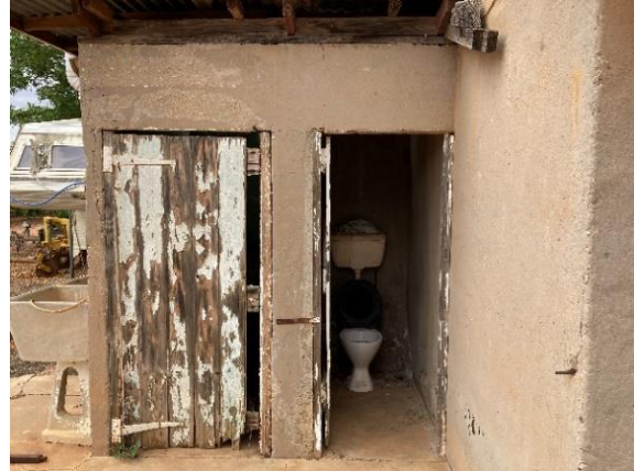
Ablutions block, toilet and shower.
