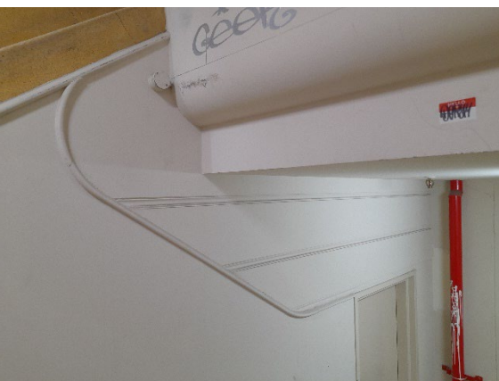
Remnant fibrous plaster decoration in western stairwell at basement level.
