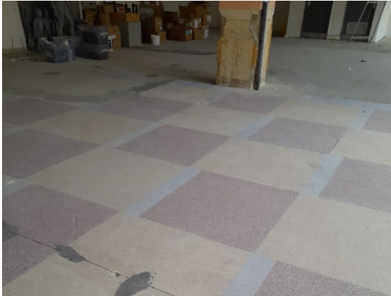
Remnant terrazzo to first floor.
