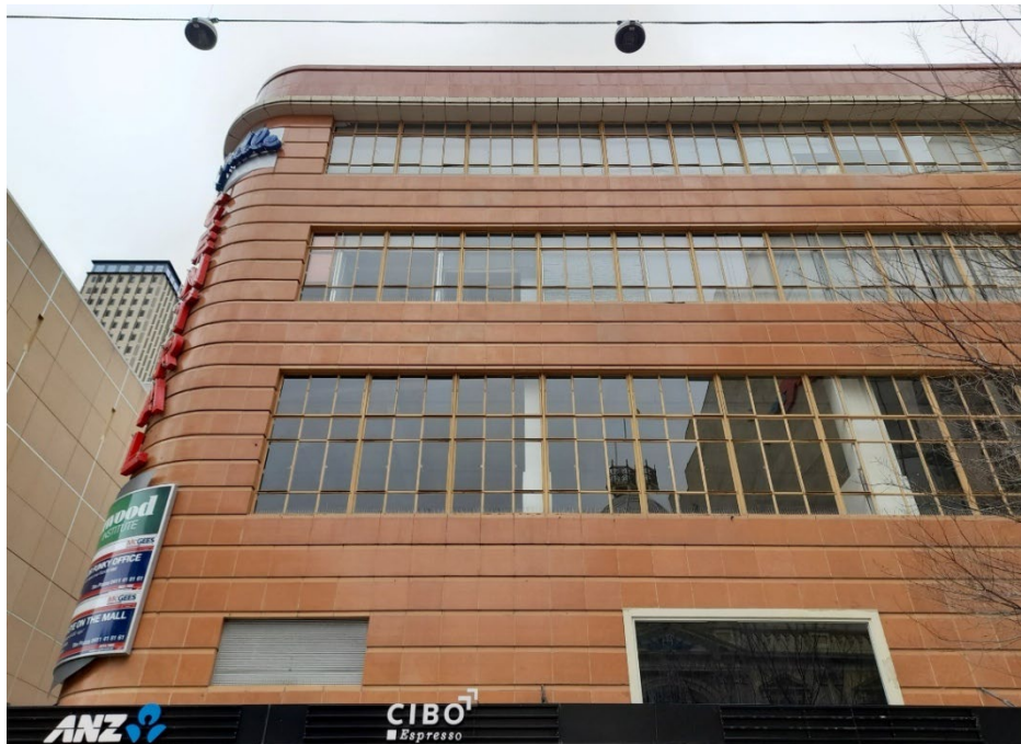
Southern elevation, note wide spans of ribbon window openings with structural columns behind (columns boxed out with non-original fabric).
