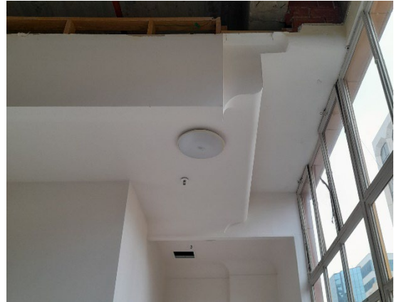
Remnant fibrous plaster ceiling coving to first floor.
