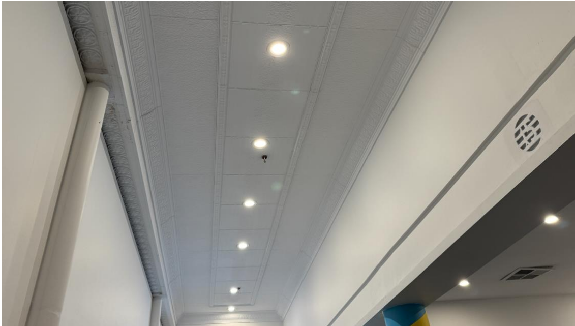
Figure 19 – Remnant second floor pressed metal ceilings and bulkhead detail
