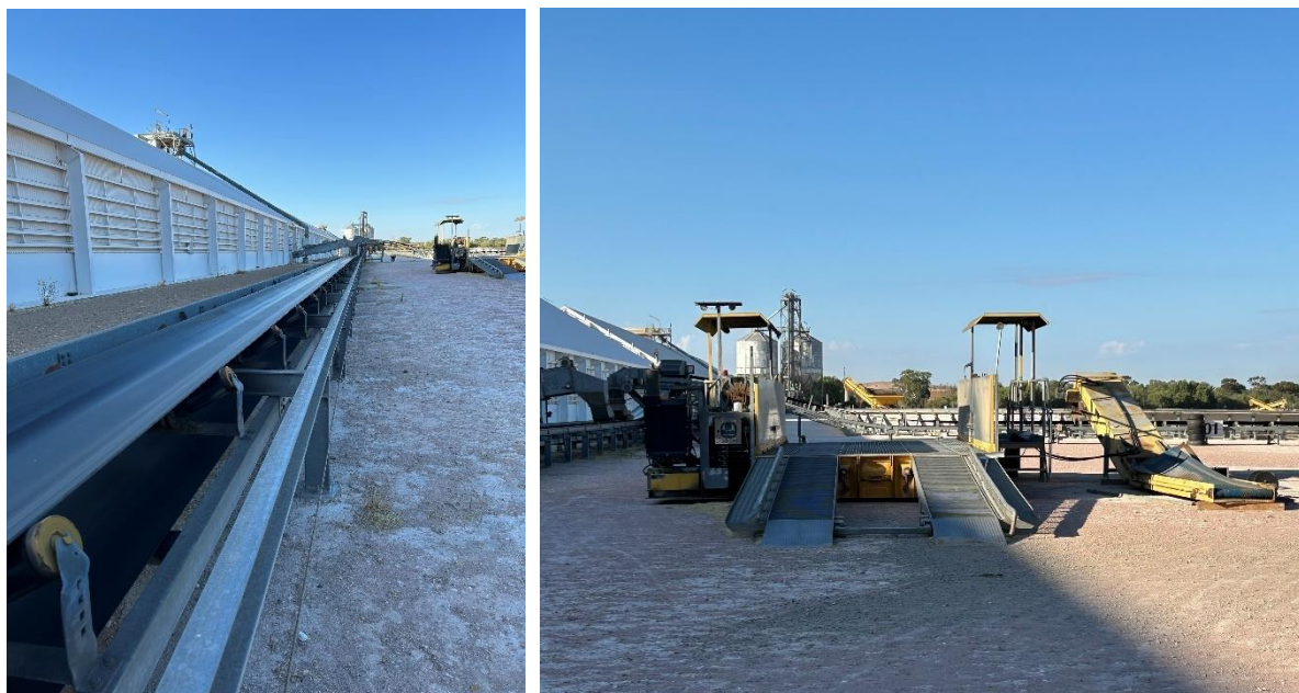
Belt conveyor along western side of paired sheds connecting storage to railway outloading bins (left) and a drive-over-hopper (right).
