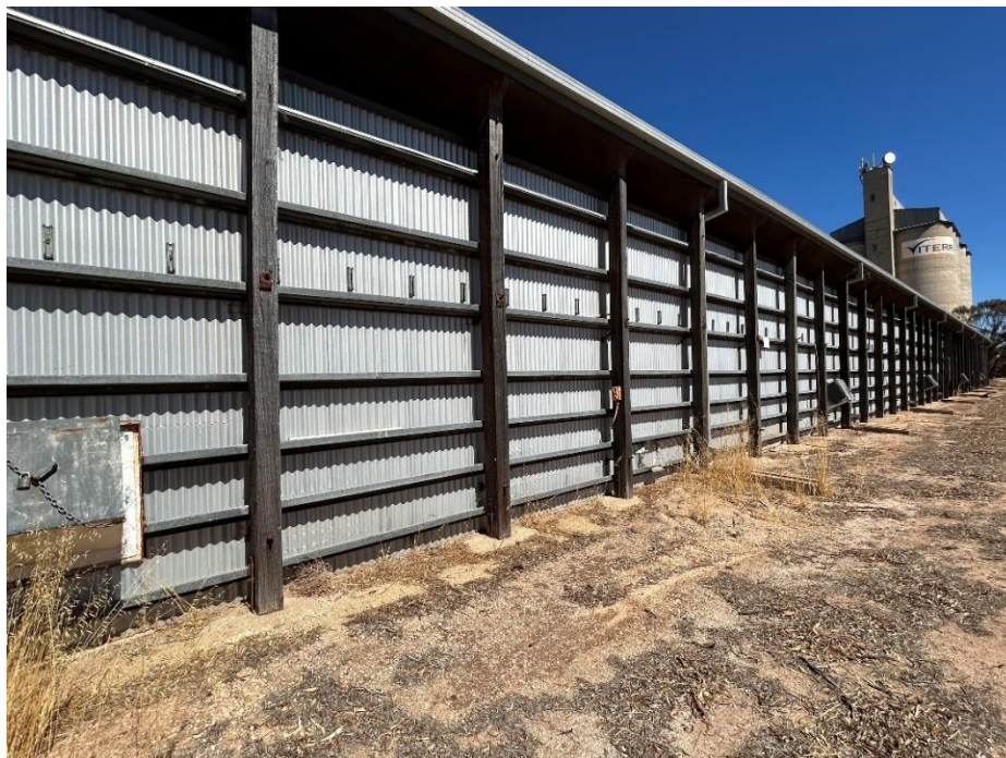
Northern elevation of the horizontal shed silo showing the building's timber and steel external structure.
