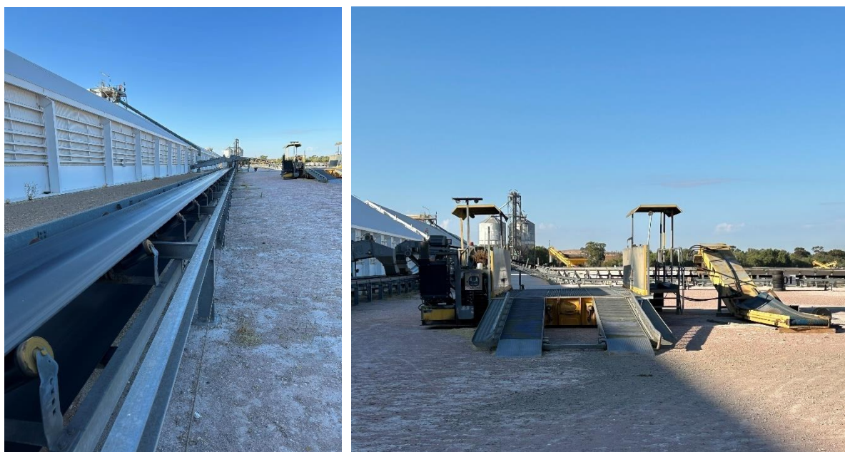
Belt conveyor along western side of paired sheds connecting storage to railway outloading bins (left) and a drive-over-hopper (right).
