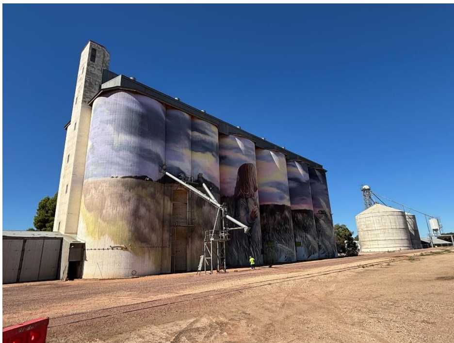
The southern concrete vertical silo with the steel vertical silo in the background.
