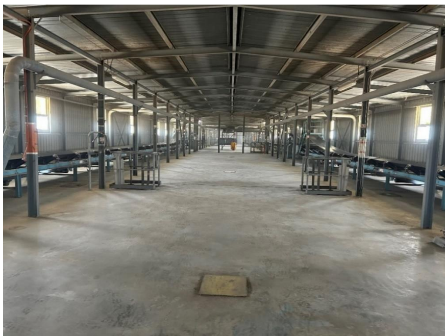
Interior of the grain conveyor enclosure at the top of the concrete vertical silo. The conveyor belts on either side feed the grain from the elevators into their allocated storage cell below.
