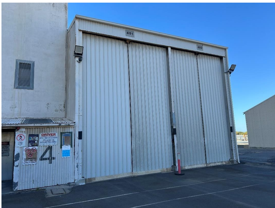
The receival hopper enclosure and base of the grain elevation of the 24-cell concrete vertical silo.
