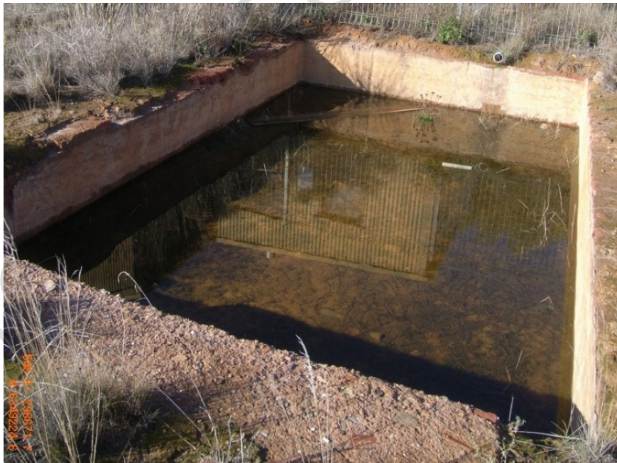
One of five in-ground tanks.
