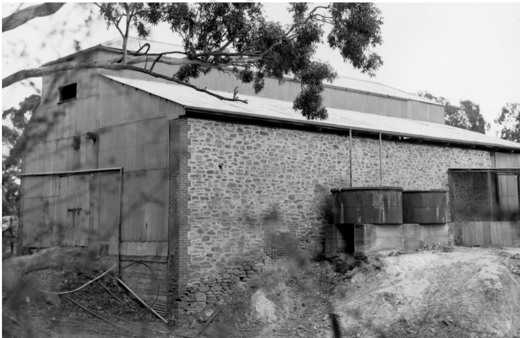
Store, probable former battery building (built c.1889), note rising damp in corner, March 1985.
