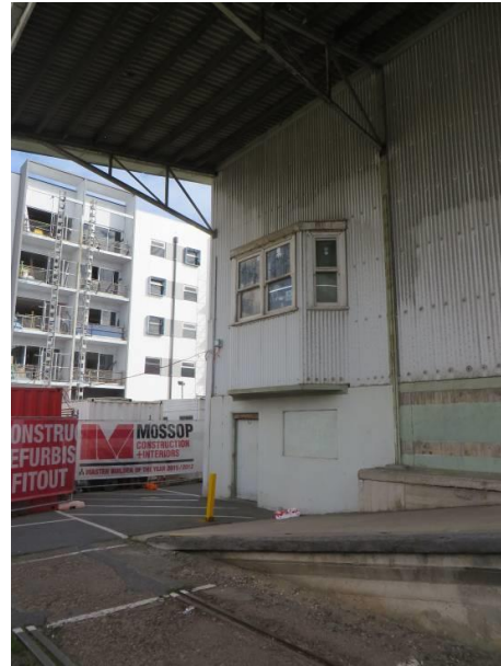
Photo 4: South west corner of Cargo Shed No. 1, showing remnant bay window, originally into the elevated tally clerk's office (now demolished). (Stephen Schrapel, 2016)
