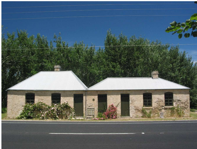
Image: The Bush Inn following conservation works, including repointing, 2003. Source DEW files.
