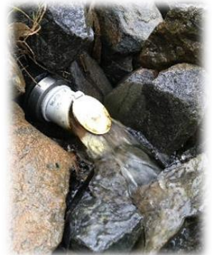
Image above. Outlet point where low flows are released into their natural flow path.
