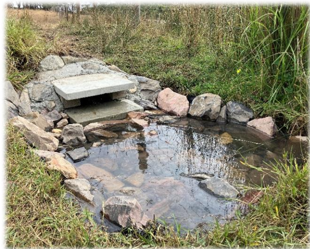
Image above. Outlet point for low flows with rock protection to prevent scouring and erosion. Image left. Device fencing option.
