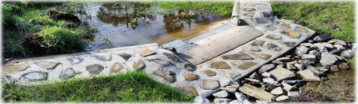
Image above. The inlet of a gravity low flow device.
