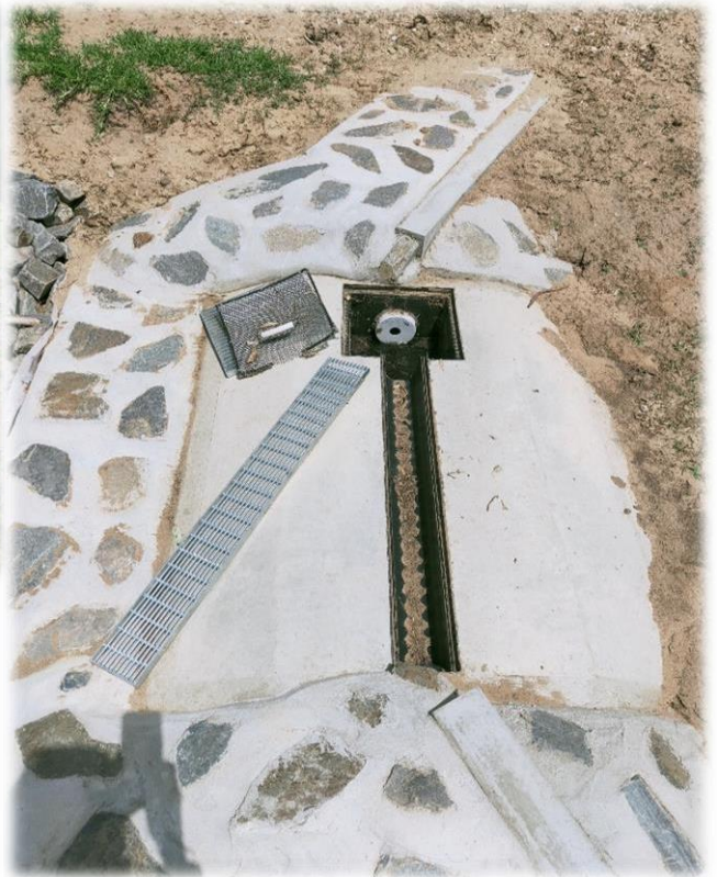
Image above. A grated gravity inlet device with sump and orifice set into the pipe system.
