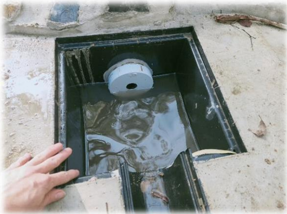
Image above. Capturing inflows via a grate and sump, a small portion (low flows) passes through the orifice into a pipe.
