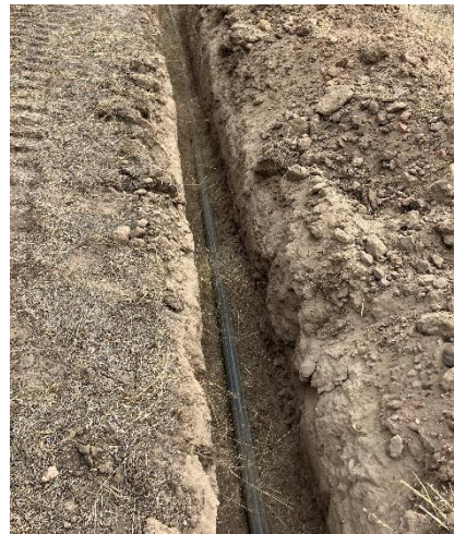
Image above. Water travels around the dam via a trenched pipe to an outlet point.
