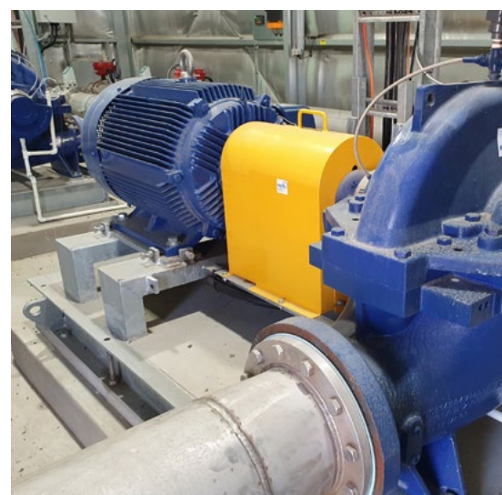
BIL pump station
