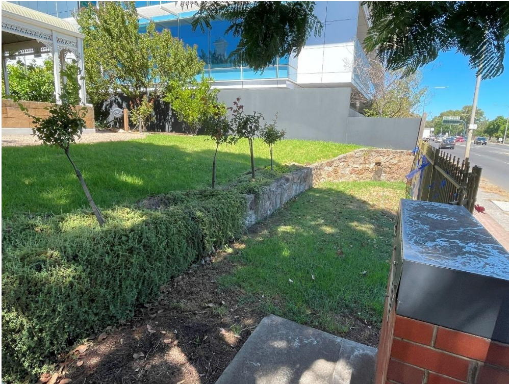
Portion of masonry retaining wall to the west of the site (adjacent to Jean Rouse Villa).
