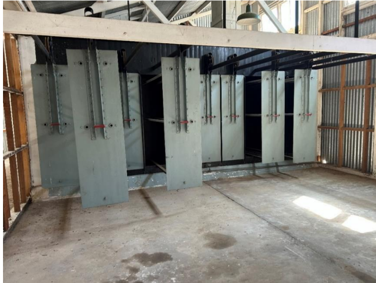
Drying cabinet in the laundry block.
