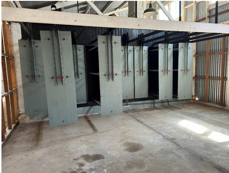
Drying cabinet in the laundry block.
