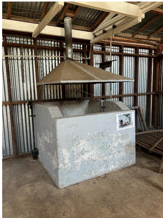
The linen steriliser located in the laundry block.
