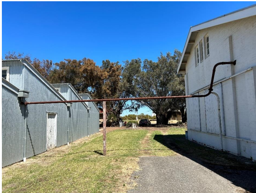
Elevated steam pipe between the boiler house and luggage store.
