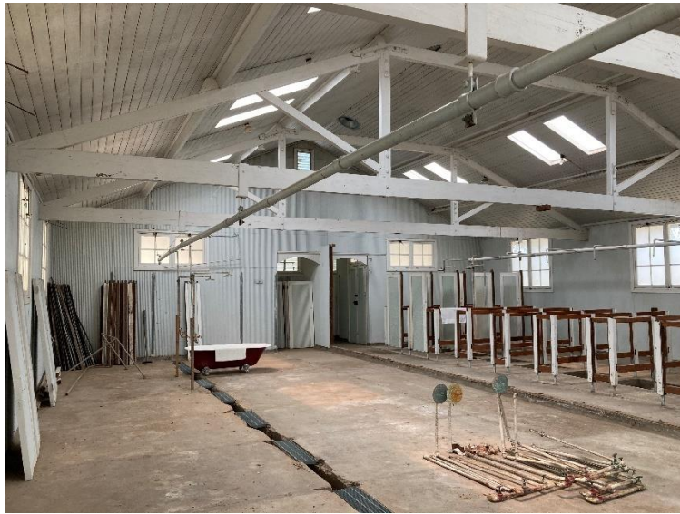
Interior of the bathing block. The cubicles were removed when the human quarantine station closed.
