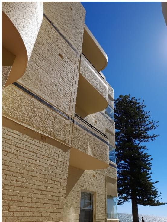
Reconstructed (new) balconies and balcony hoods, note wall transition and new vertical structural member
