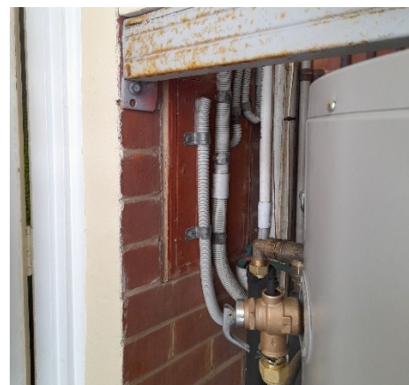
Hot water service penetrating original service hatch
