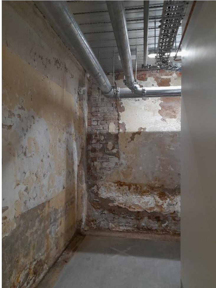
Rising damp damage in the basement.
