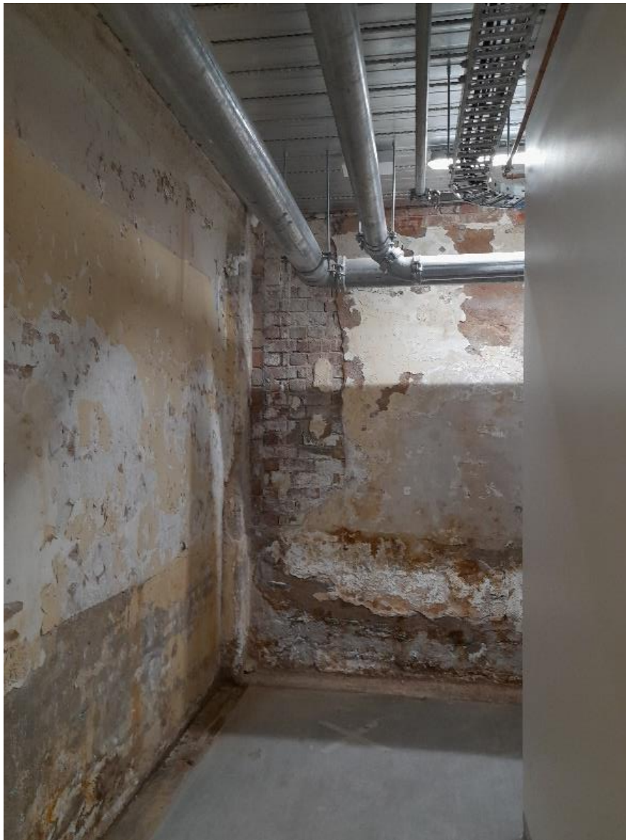
Rising damp damage in the basement.
