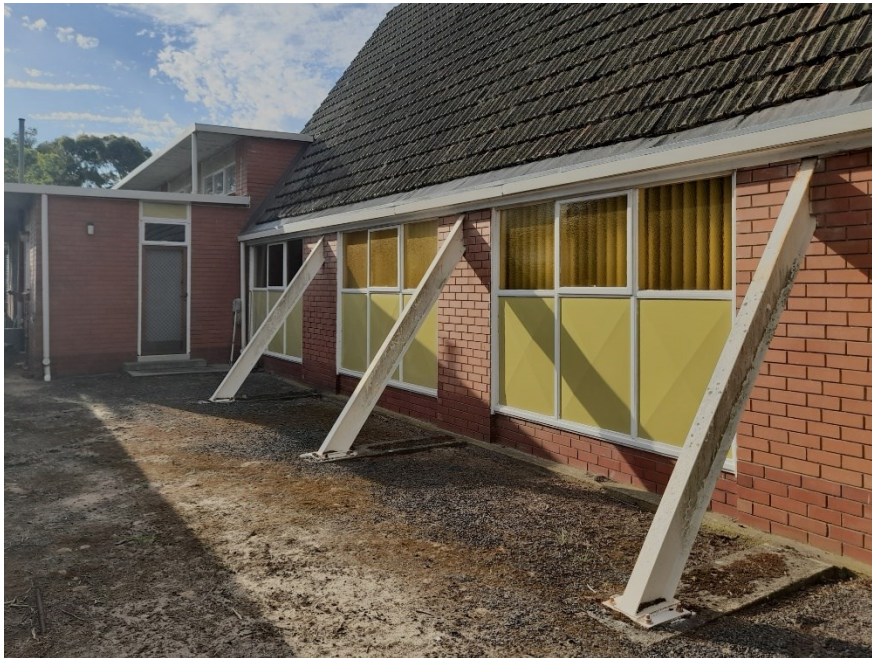
Southern side of chapel showing rolled steel 'buttresses' and 'Porcipanel' spandrels, 30 September 2023
