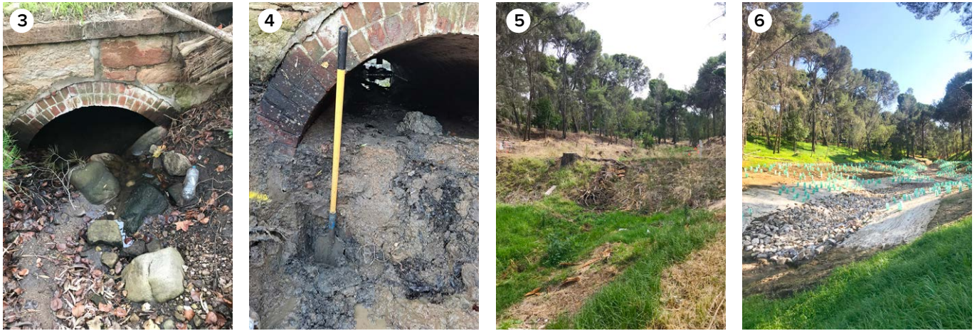
1. Erosion hole at base of dam wall with water seeping through. 2. Erosion hole at top of dam wall – this was being used as a crossing point by walkers and riders and causing safety concerns. 3. Downstream by the historic drain outlet which was blocked by sediment build up. 4. Shows depth of sediment build up that was blocking the drain. 5. Before: Looking upstream at failed dam wall, pine trees removed. 6. After: Looking upstream, where the dam wall was removed and replaced with rock chutes, jute matting installed, planting and hydro-mulch completed.
