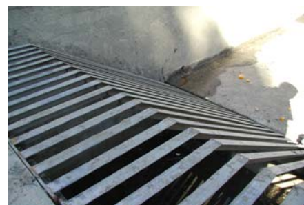
Litter is pushed down the screen, thus leaving the gaps free for water to flow through it.
